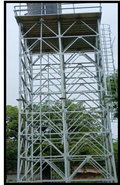
12 M STRUCTURE — ACTUAL JJM INSTALLATION, GORDHA (CHHATTISGARH)
